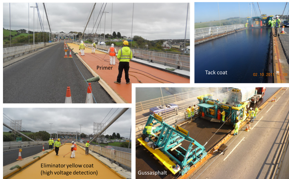
FIGURE 6. The Implementation of rehabilitation work in 2011 at location 125 m ahead of the toll gates
