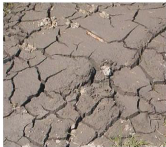
FIGURE 2. Feature of cracks on expansive soils during swell-shrink cycles
