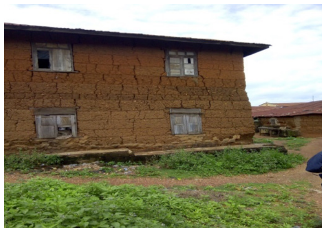
FIGURE 2. Typical building showing dilapidated wooden windows
