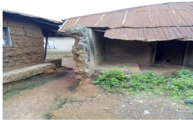
FIGURE 1. Typical building showing collapsed mud wall and eroded foundation
