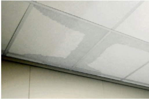
FIGURE 3. Dampness effect clearly be seen at this ceiling due to leakage from the wet area above
