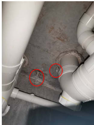
FIGURE 4. Leakage of toilet detected on the floor trap (down pipe)
