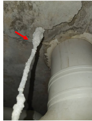
FIGURE 5. Calthemite formed from concrete
