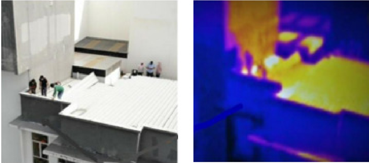
FIGURE 5. Rooftop area and infrared thermographic imaging at Locations 1 and 2
