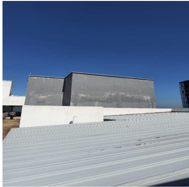
FIGURE 4. Metal roof at the rooftop were dismantle to test dampness at Location 1 and 2
