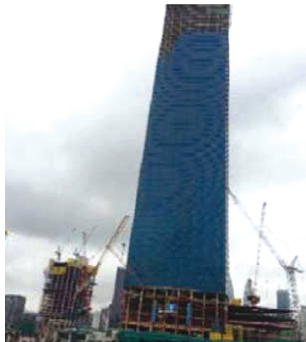
FIGURE 1. A photo of The Exchange 106 or previously known as TRX Signature Tower during construction taken on 2 November 2017 (KLCC at the back of this structure)
